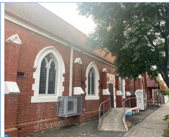
View from south of south elevation of showing fenestration. Source: Extent Heritage Pty Ltd, 2024.
