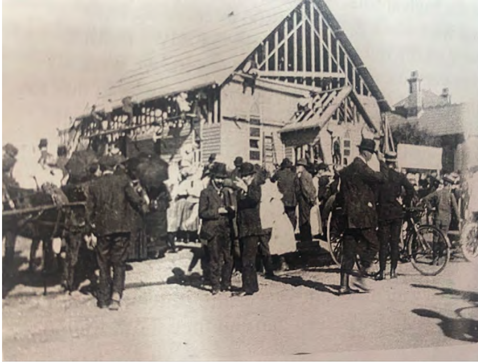
Figure 2 Photograph of the construction of the original Preston Church of Christ, constructed in a day on 25 March 1911. Source: Nancy Garth (Ed.). Preston Church of Christ Book of Memories.
