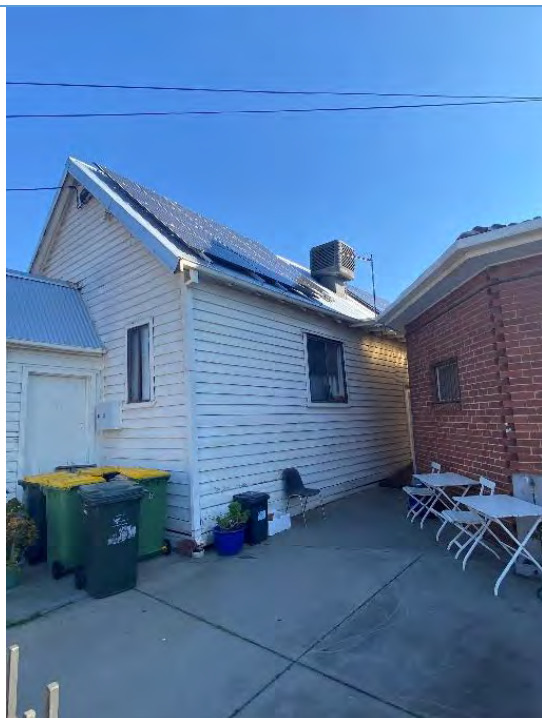
Oblique view of the Church Hall's northern elevation. Source: Extent Heritage Pty Ltd 2024.
