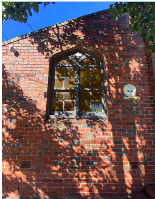
View of façade of Former Church of Christ, Preston from north. Source: Extent Heritage Pty Ltd.
