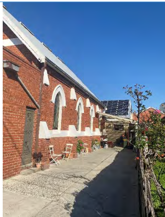
Oblique view of the Church's western elevation. Source: Extent Heritage Pty Ltd 2024.
