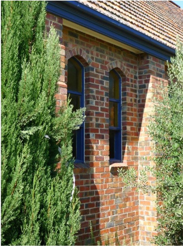
Figure D6. Clinker brick walls, buttresses, pointed arched windows and window sills. Narrow three light timber windows.
