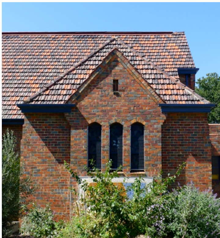
Figure D5. The west elevation facing Gillies St has a deeply sculptured design with pointed arches, buttresses, which are more typical of traditionalist Gothic churches.
