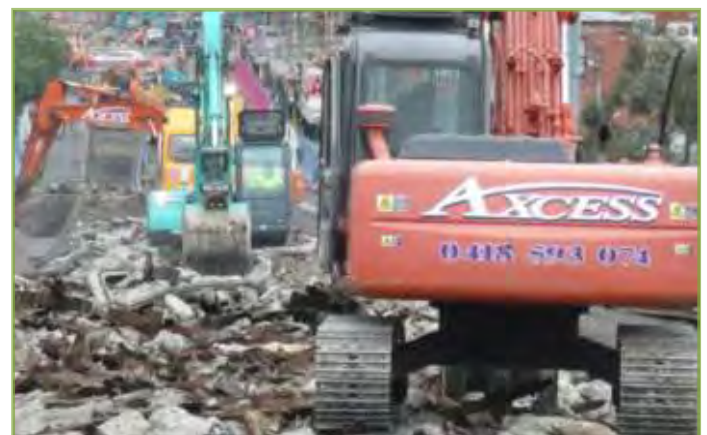
High Street Northcote Tram Works - Phasing Works is Critical to Minimise Prolonged Disruption Image: Outlines Landscape Architecture
