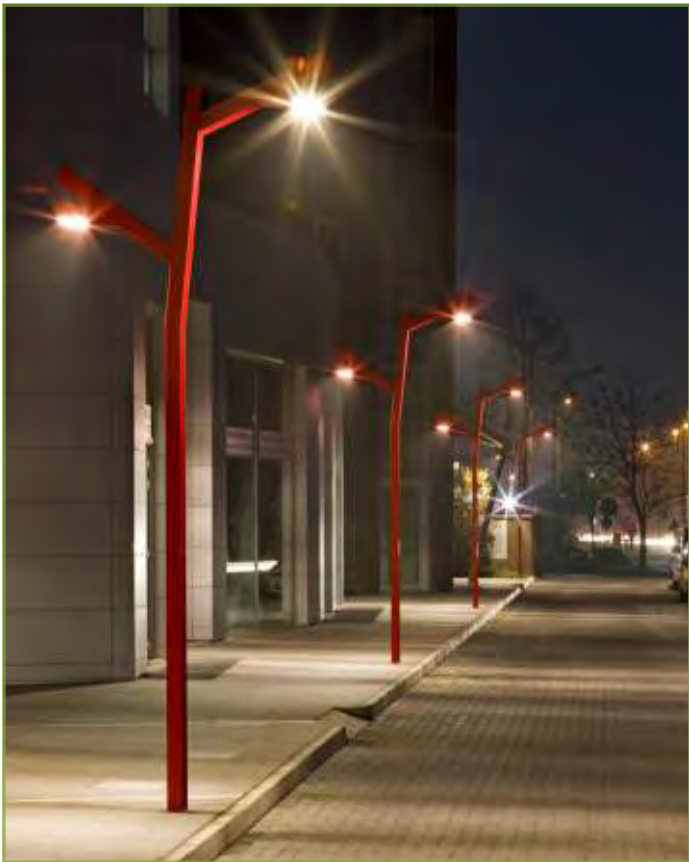
Enhanced Street Lighting - For Nighttime Activation, Enhanced Amenity & Accessibility Image: fontanaarte.com
